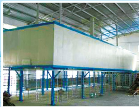
吊栏烘干线 Suspension bar drying line
